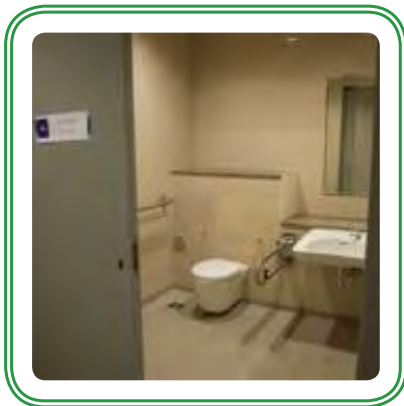
Toilet Disabilitas Disability Toilet
