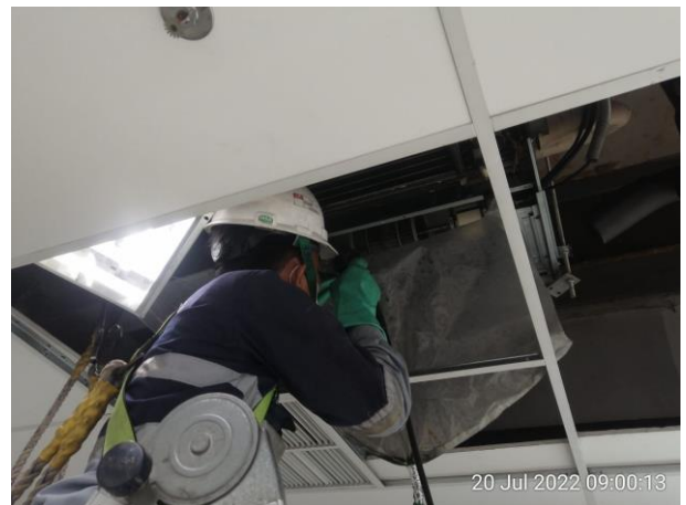
Cleaning unit Air Conditioning System
